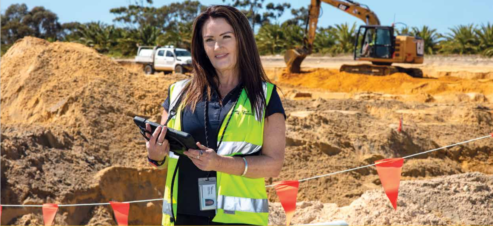
The City's Sand Drift Compliance Officer, Heather Sheehan, at a Sinagra development site.
